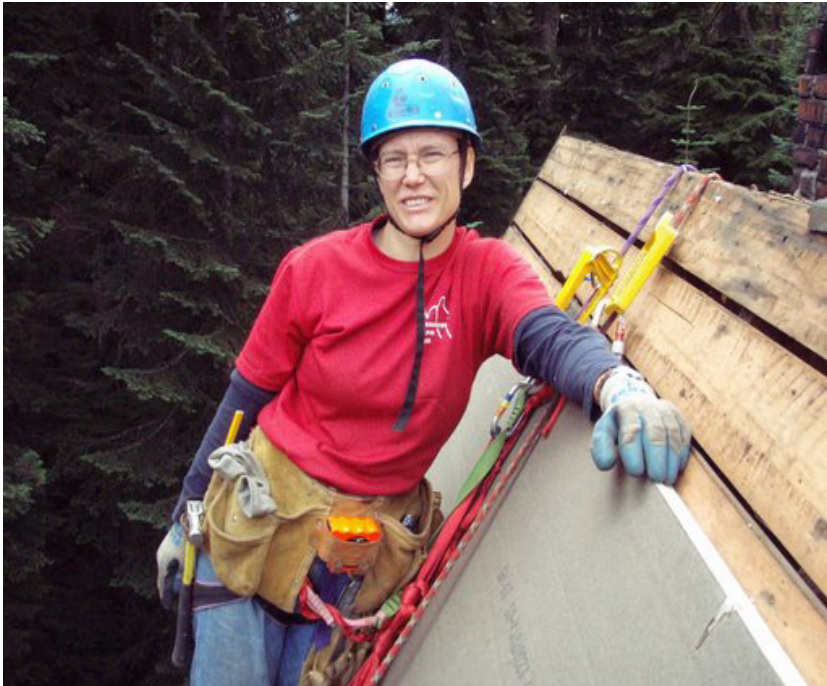
Eli Holmes on the gentleman's dorm putting down the insulation. Eli was able to put in the full 12 hours days and still take all these pictures!
